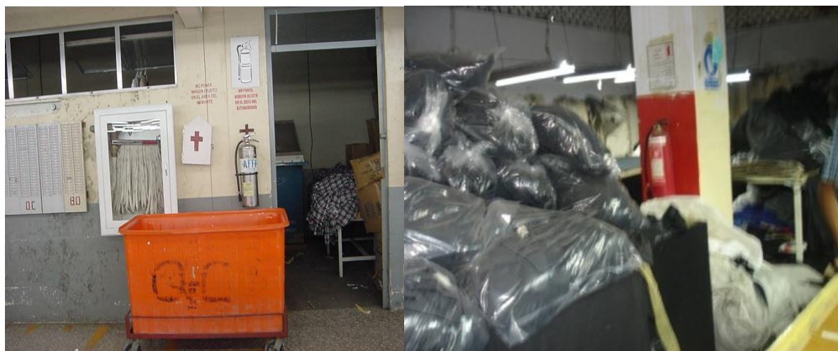
(Example: Blocked fire extinguishers)
