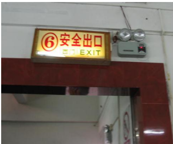
(Example: Emergency exit properly marked)
